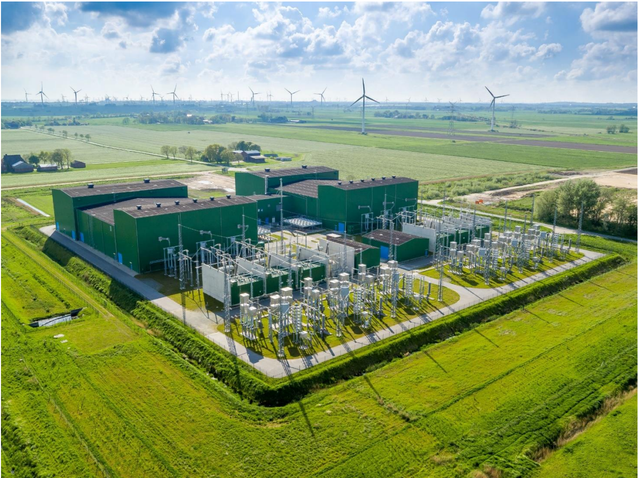
Figure G.4: NordLink HVDC converter station
