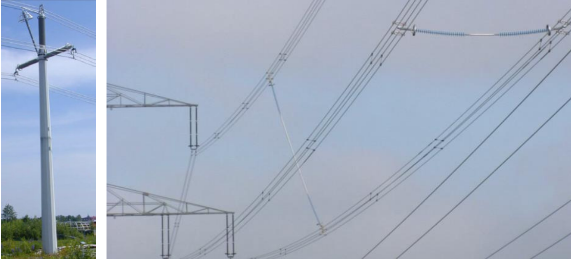
Figure D.23: a) 420 kV line in Norway, b) Inter-phase spacers
