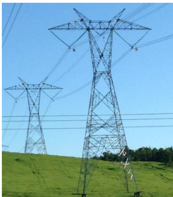
Figure D.27: Western Alberta 500 kV transmission line
