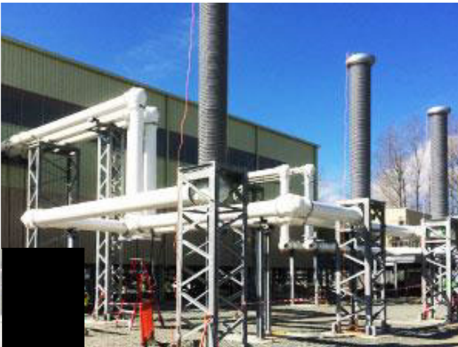
Figure H.9: SF 6 -free GIL installation at a National Grid substation
