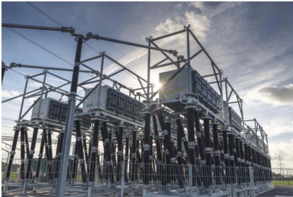
Figure H.3: SSSC Installation by Smart Wires at NGET's Penwortham substation
