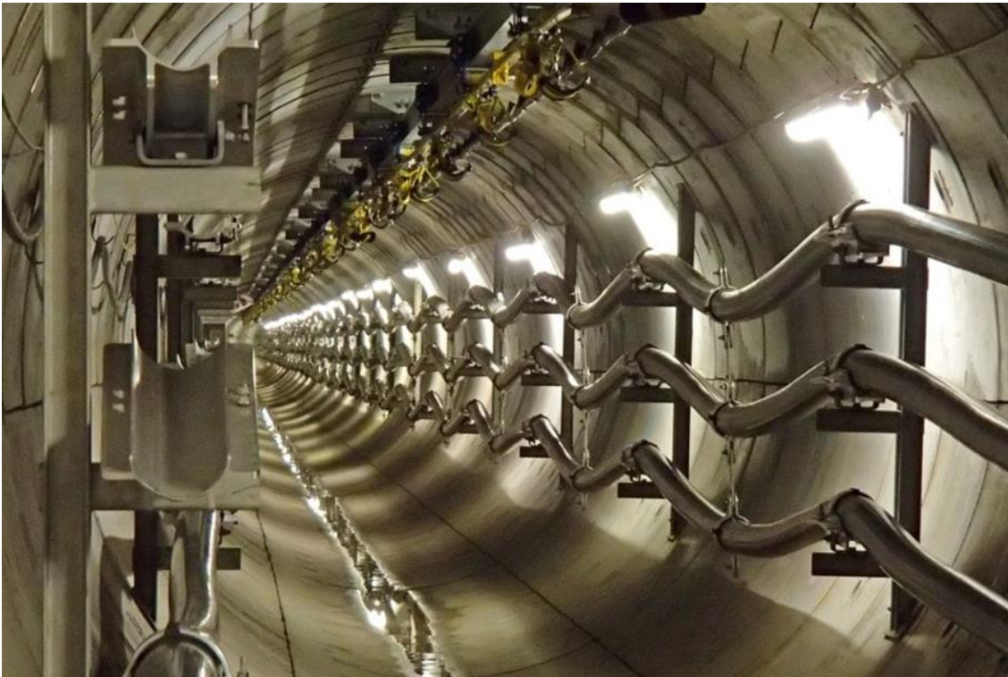
Figure F.4: Cables installed within a tunnel system
