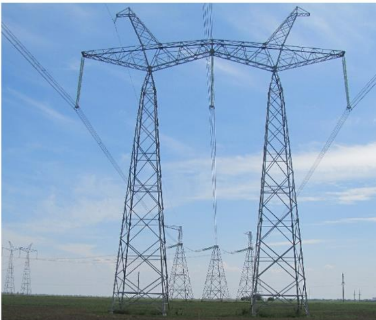
Figure D.26: 750 kV Zaporizhzhia NPP – Kakhovska OHL, Ukraine
