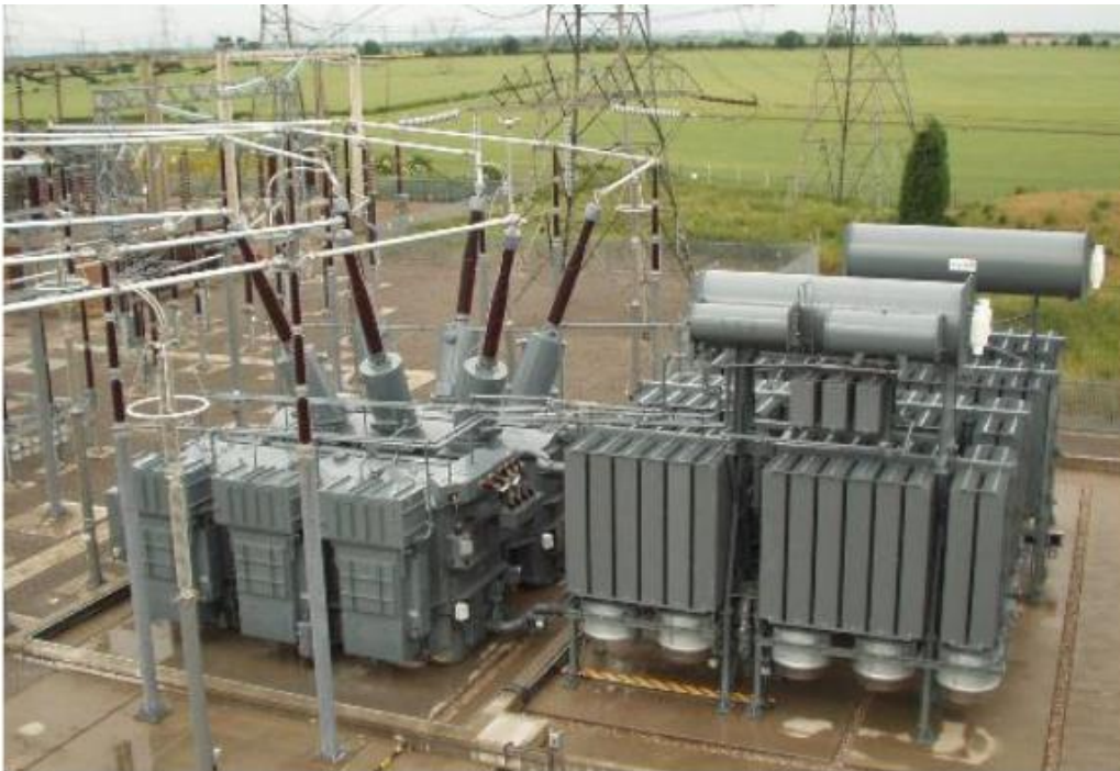
Figure H.4: Example of a quadrature booster at NGET’s High Marnham substation
