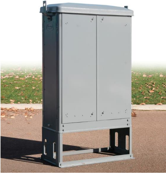
Figure E.3: Example of above ground link pillar
